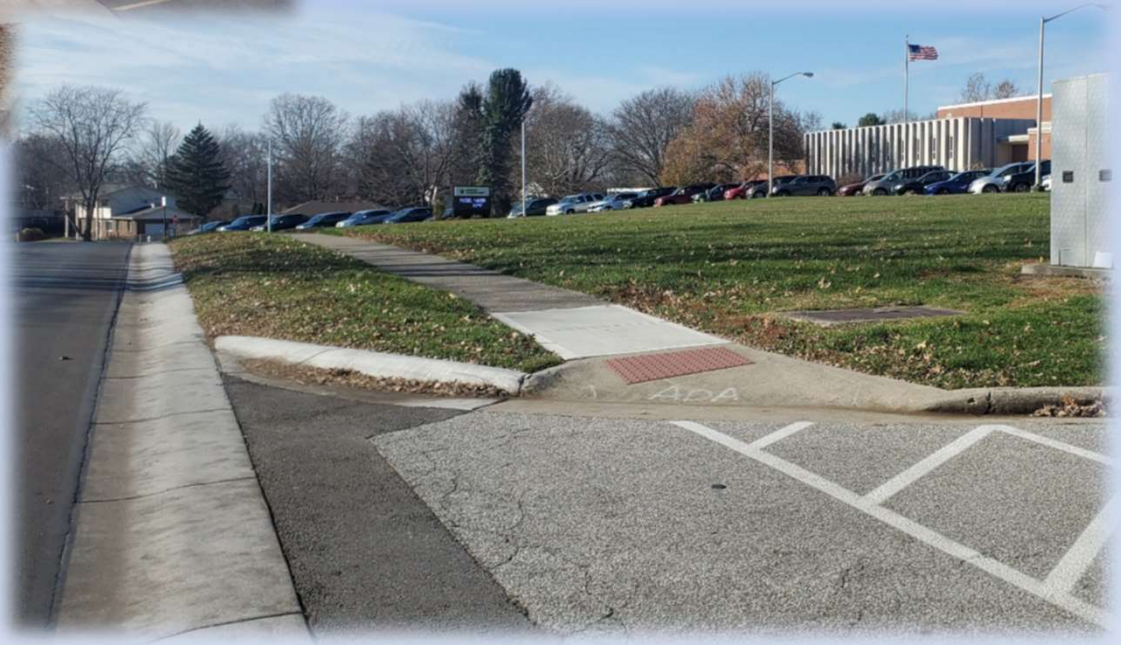
Replaced deteriorated sidewalk blocks around the school and installed lower curb for possible future school related improvements along Northport
